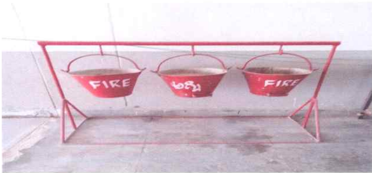
Fire extinguishers for safety
