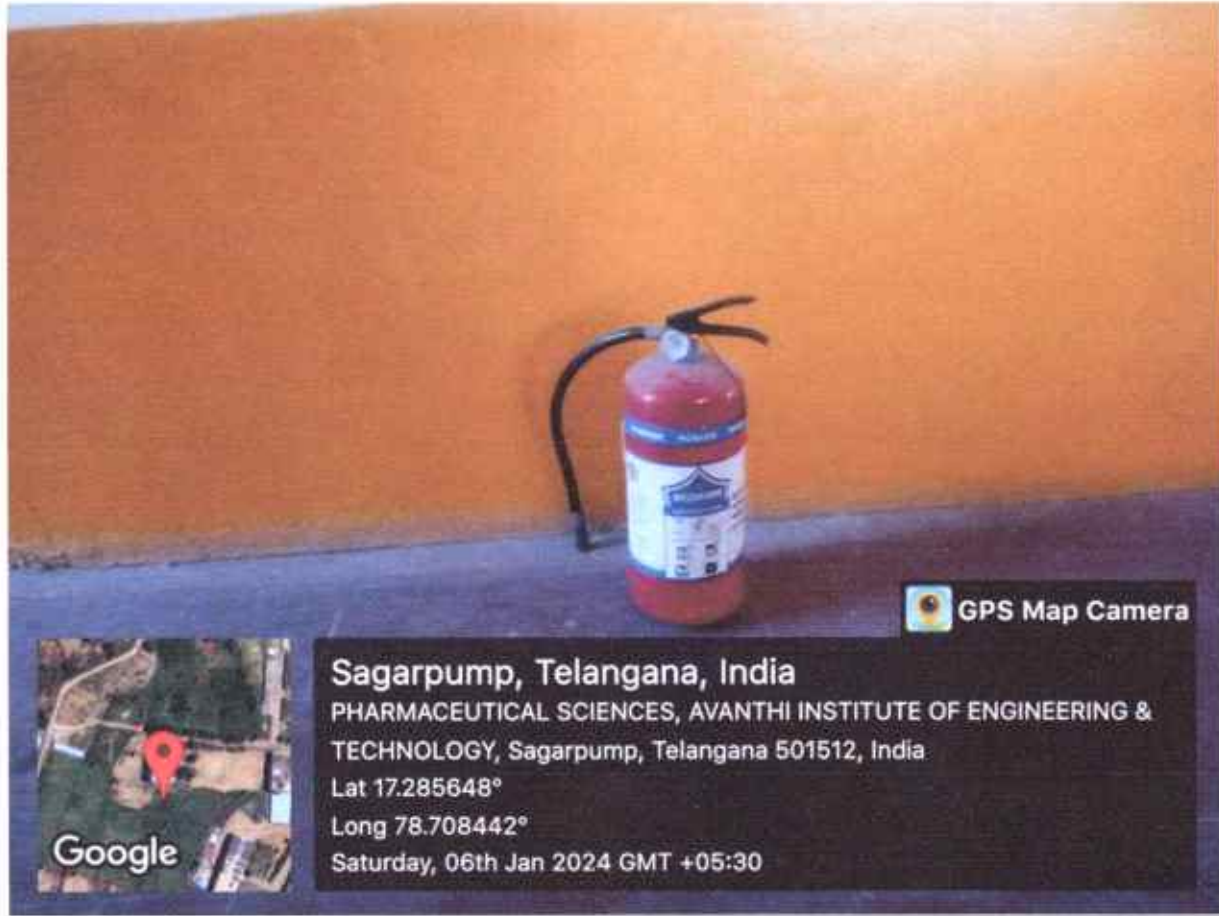
Fire extinguishers for safety
